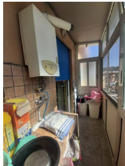
Scaldacqua a gas collocata in veranda
